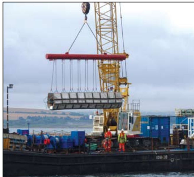
Protective matting for the new outfall pipe is lowered into the Forth.
